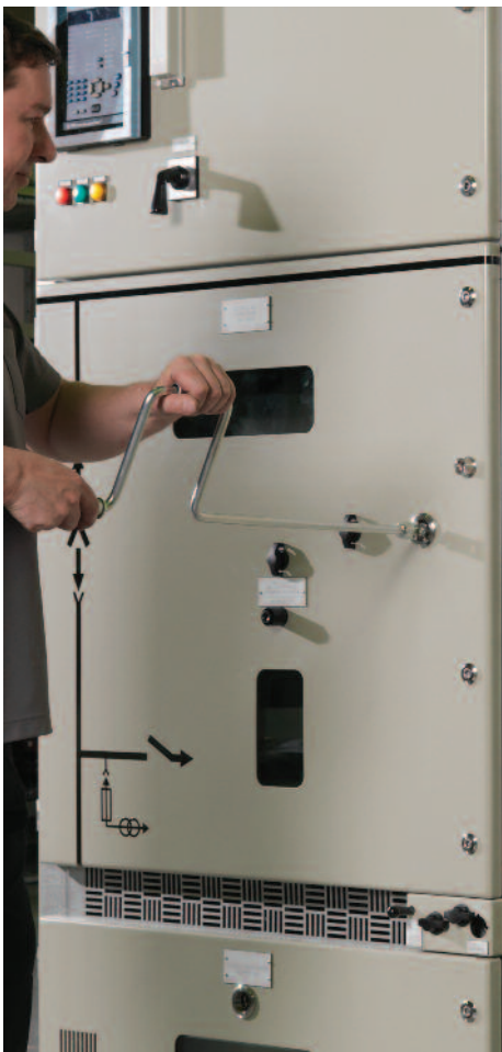
Fastening Circuit Breaker Compartment Door
