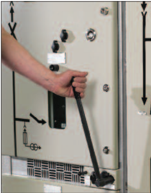
Operating Circuit Earth Switch
