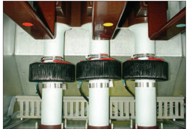
CTs mounted on earthed-screen bushings
