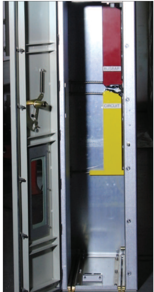
VCU Cubicle Showing Shutters and Guide Rails
