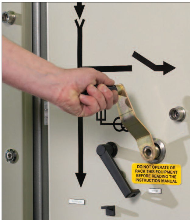
Racking VCU Behind Closed Door
