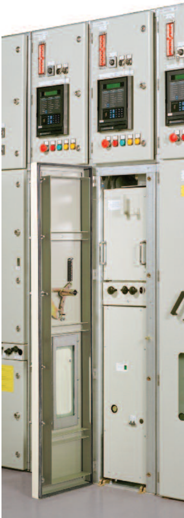
Withdrawal of Vacuum Contactor Truck
