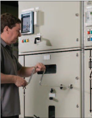
Racking Circuit Breaker
